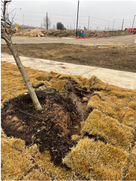
Tree not stake properly Sod poorly installed
