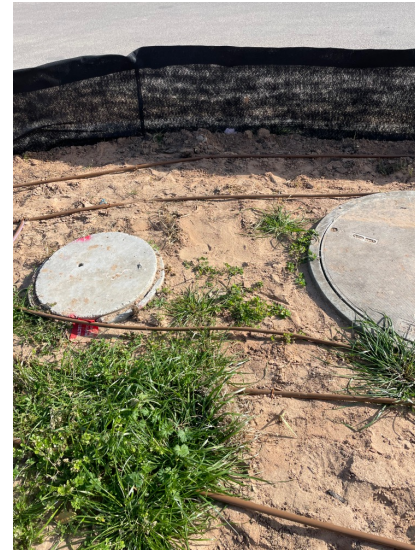
Not proper coverage; weeds
