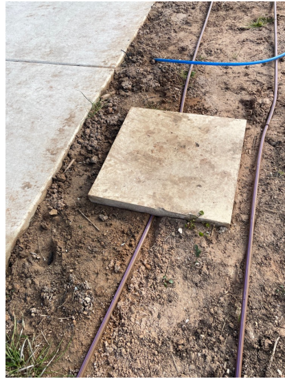
Drip under stepping-stones
